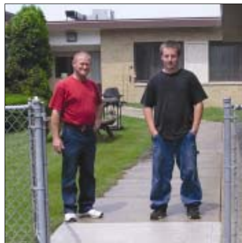
Jay Crossley and Steven Creeden stand on the wheel chair ramp that Jay worked on.
